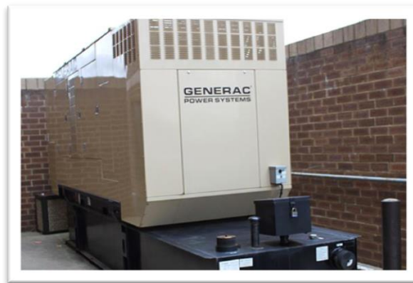
Commercial generator. Credit: Dwight Burdette
